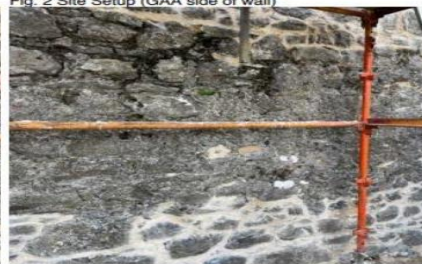
Fig. 4 Area of wall not repointed as repointing is intact in this area
