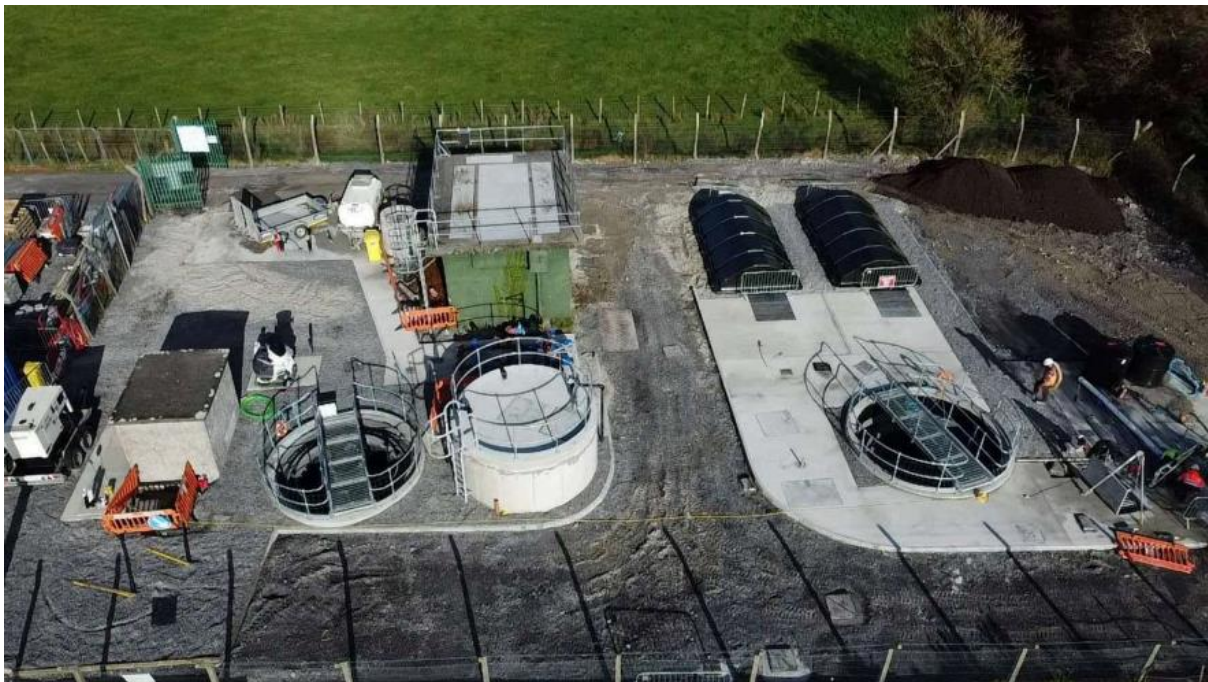
Ahascragh Wastewater Treatment Plant
