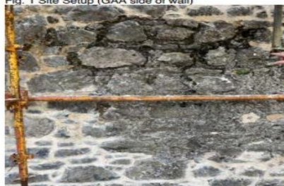
Fig. 3 Area of wall not repointed as repointing is intact in this area
