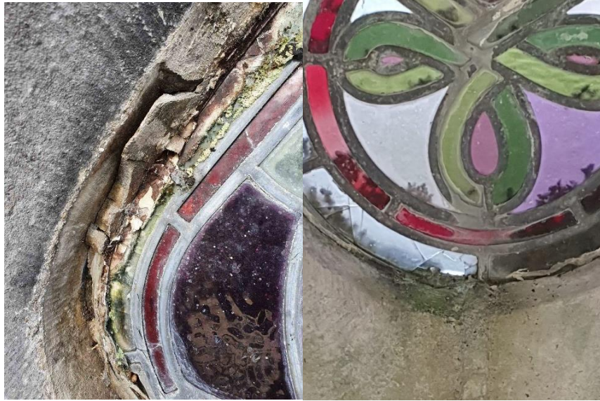
Cracked glass decayed lead comes , algal growth due to water ingress
